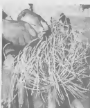
IT TAKES dexterity and a steady hand to random splice a 160-pair telephone cable.
